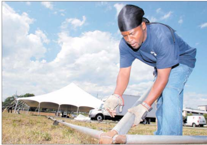
Celebrations of Columbia employee Mike Davis helps make preparations for today's groundbreaking ceremony.
